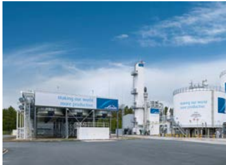
LION™ modular air separation plant at Rothenbach
