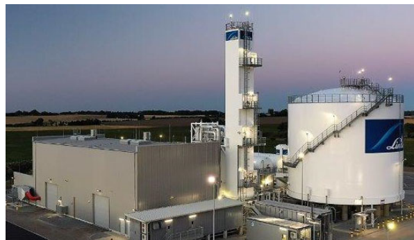
Linde Flexible Air Separation Plant (FlexASU®) in Vejle, Denmark
