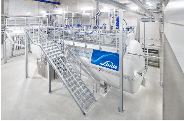
Linde Hydrogen Liquefaction Plant, Leuna, Germany
